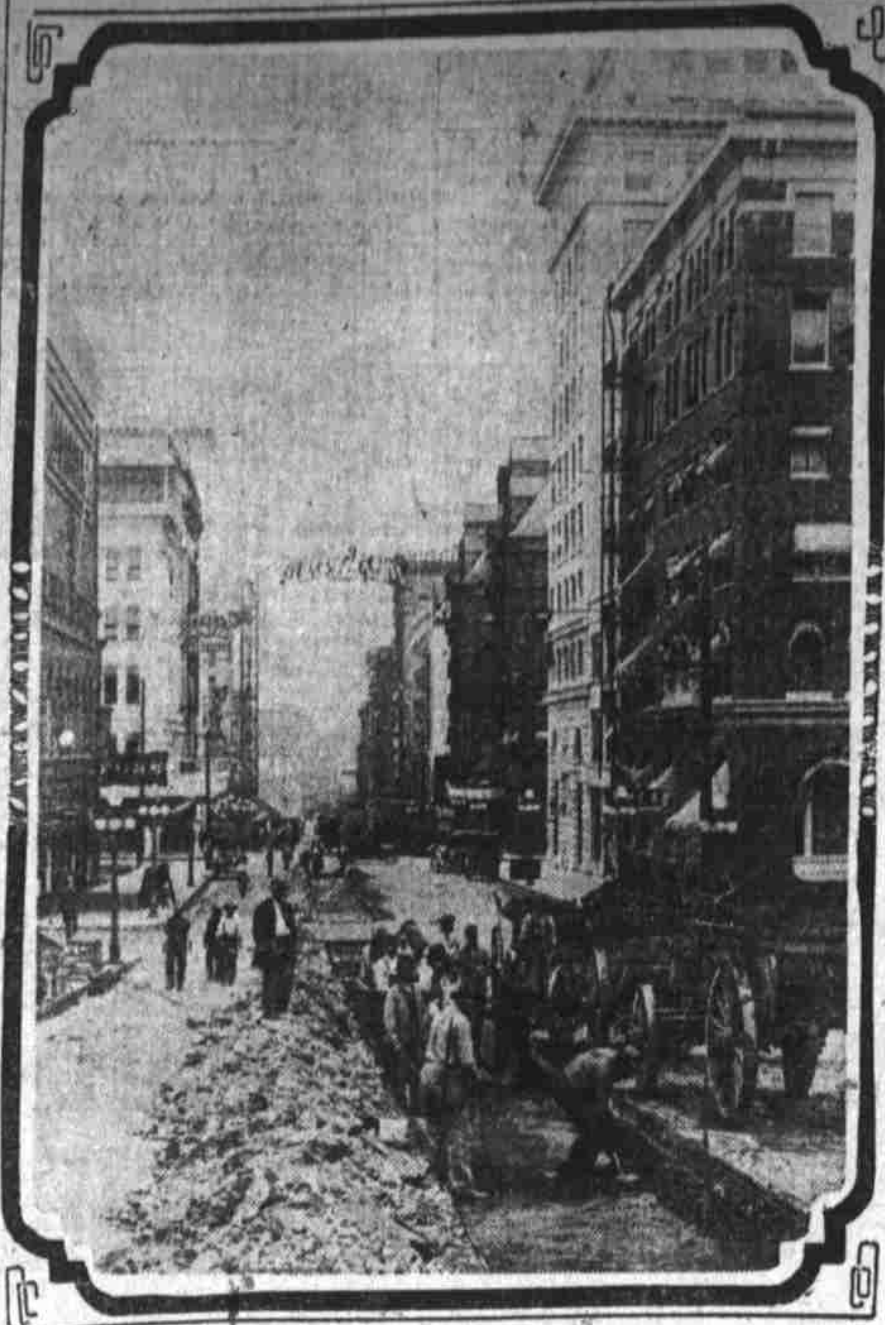
View of Broadway street, looking north, showing workmen of Portland Railway, Light & Power company tearing up pavement for roadbed of proposed new carline.
