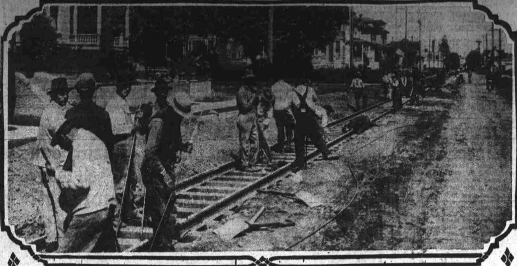
Scene on Broadway, East Side, where crew of Portland Railway, Light & Power company is laying track. Cars will be running over bridge and up to Jefferson street by September.
