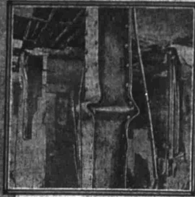
The Effect of Not Concreting Iron Columns: From the Calvert Building in Baltimore.
