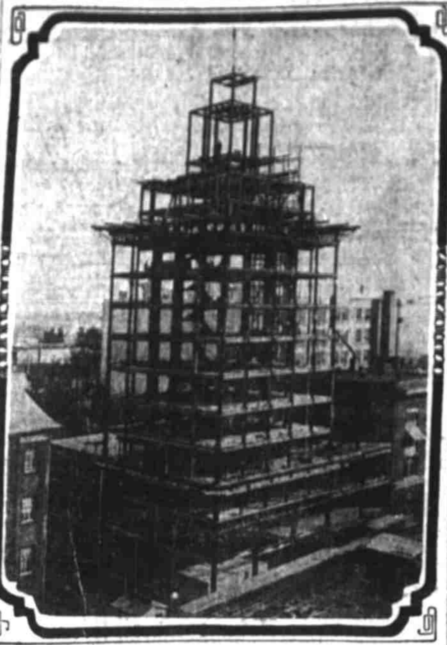
Completed steel frame of New Journal building—Rapid progress is being made in laying concrete floors, and encasing steel in concrete.
