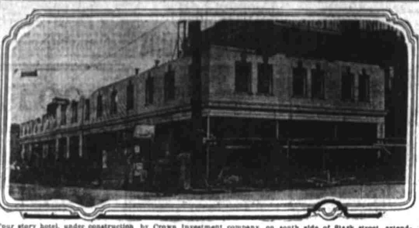
Four story hotel, under construction by Crown Investment company, on south side of Stark street, extending from Tenth to Eleventh street.
