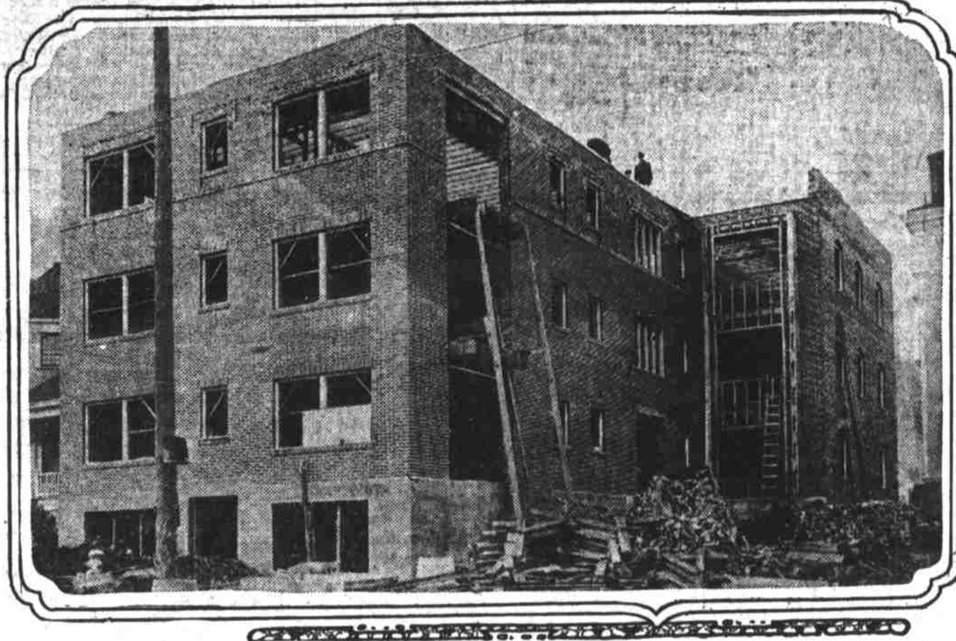
Apartments under construction at Twelfth and Harrison streets for C. C. Smith.
