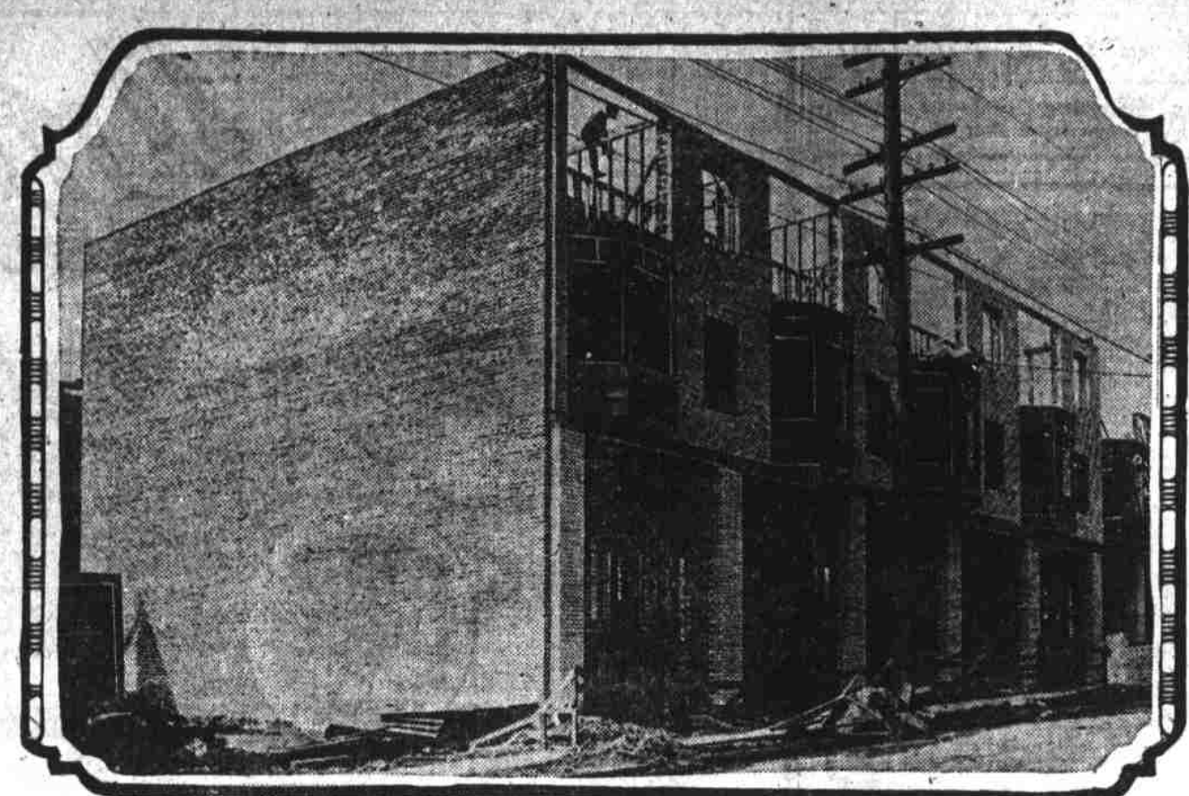
Korell-Gordon, 3-story brick store and apartment building, under construction at intersection of Morrison, Washington and Ella streets.
