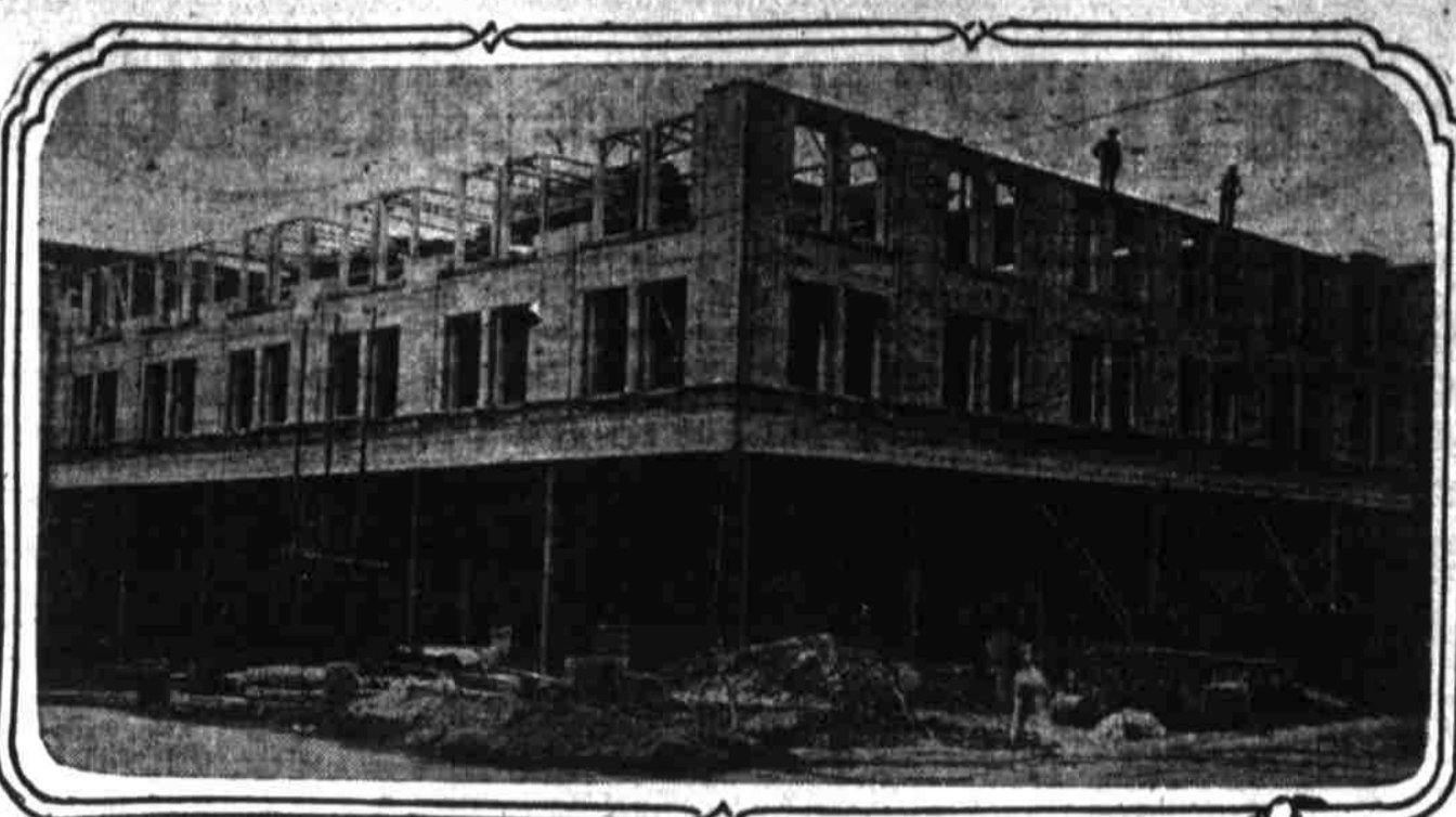
Strong building, four-story and basement business structure under construction at northeast corner of Tenth and Alder. The building will cost approximately $60,000 and has foundation of sufficient strength to carry several additional stories.
