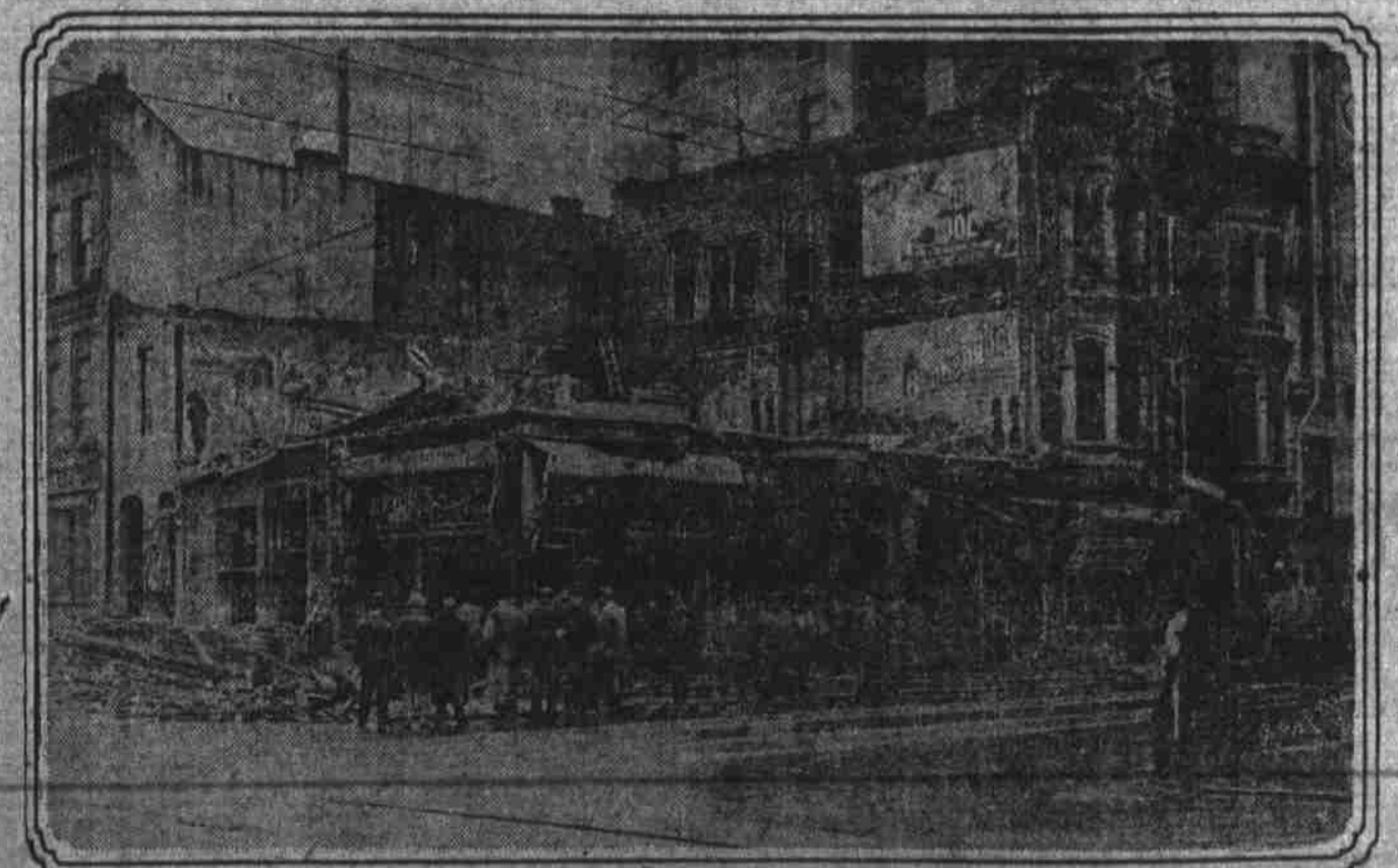
Demolishing old frame store buildings at Fourth and Washington streets to make way for 12 story office building to be erected by the Syndicate Company.
