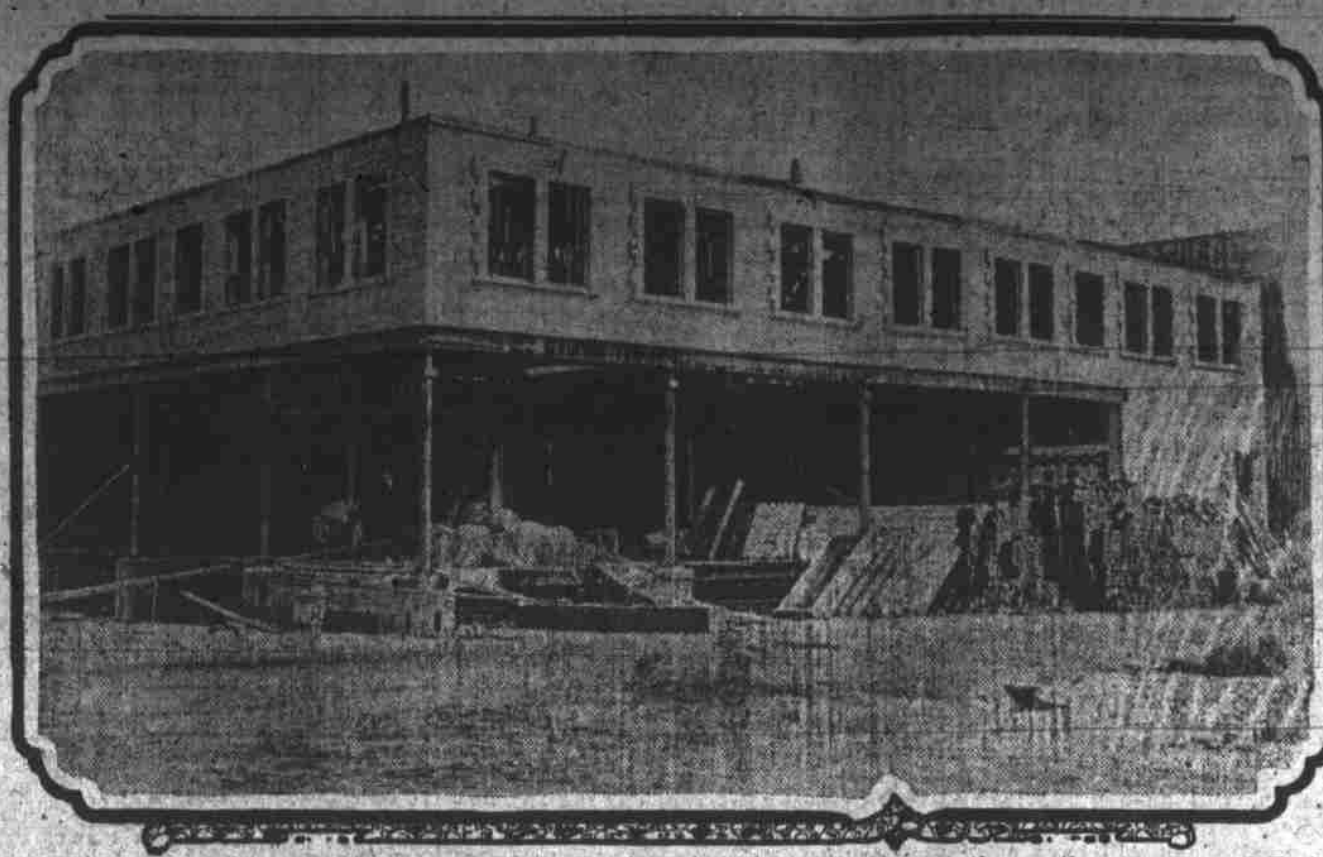
New Bakery company's new three-story brick building under construction at the northeast corner of East Seventh and Belmont streets. The structure occupies a quarter block and will cost about $35,000.
