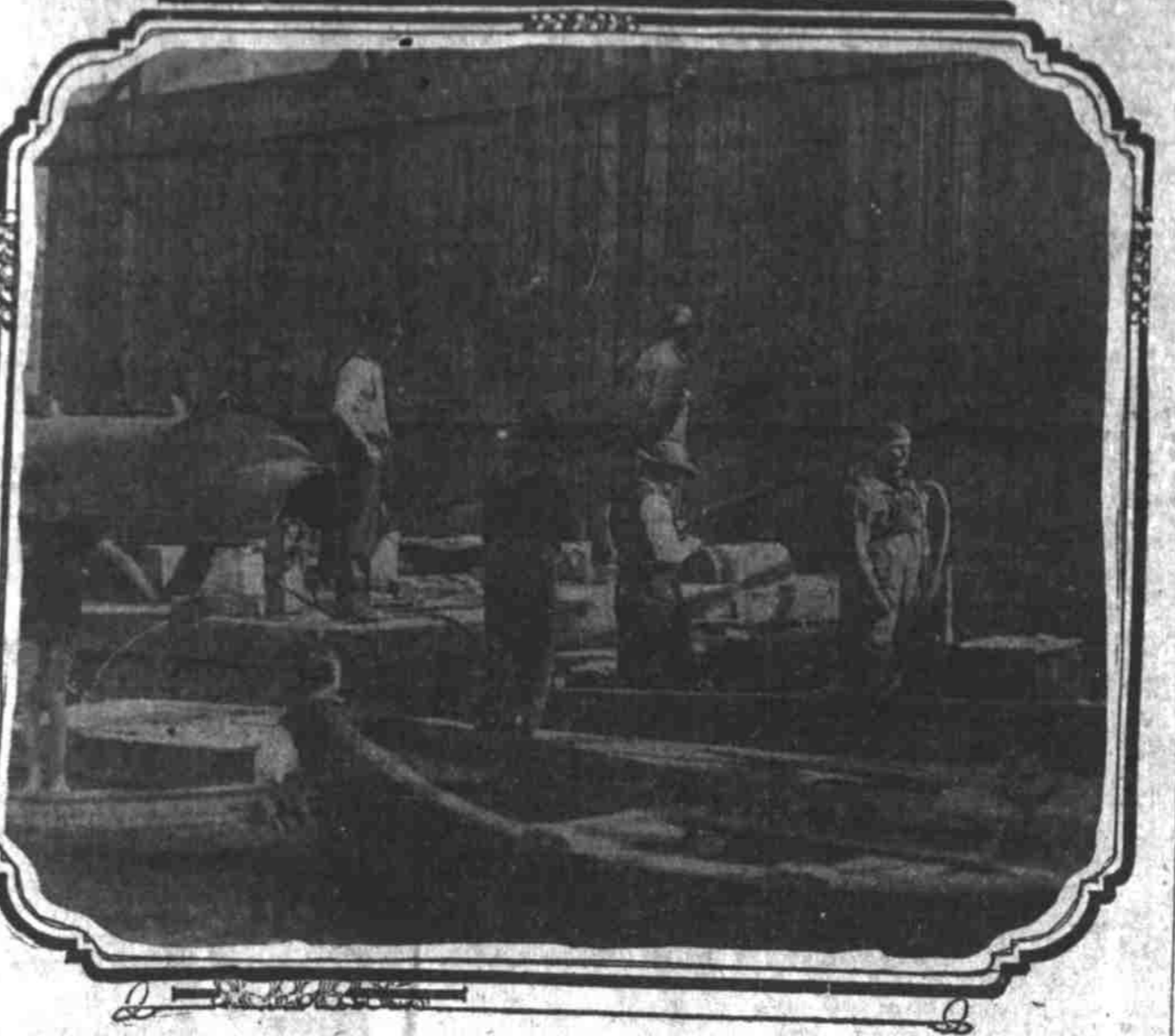
Divers began the work of clamping a huge iron sleeve over the broken water main under the Willamette yesterday morning. The under half of the big sleeve was slipped over the fractured tube and the other side of the clamp will be riveted on this afternoon.
