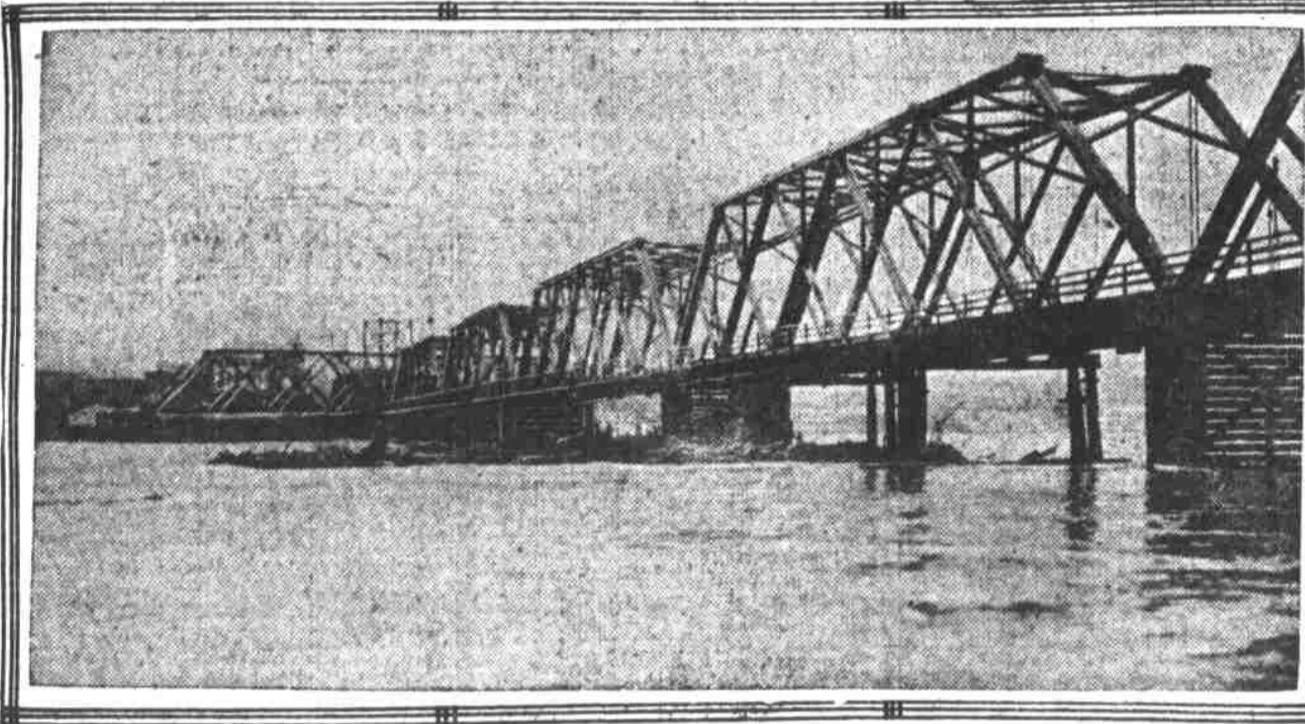
Madison Street Bridge, Portland, Showing Falsework Carried Away by Swift Current and Driftwood Piled Up Against Piers.
