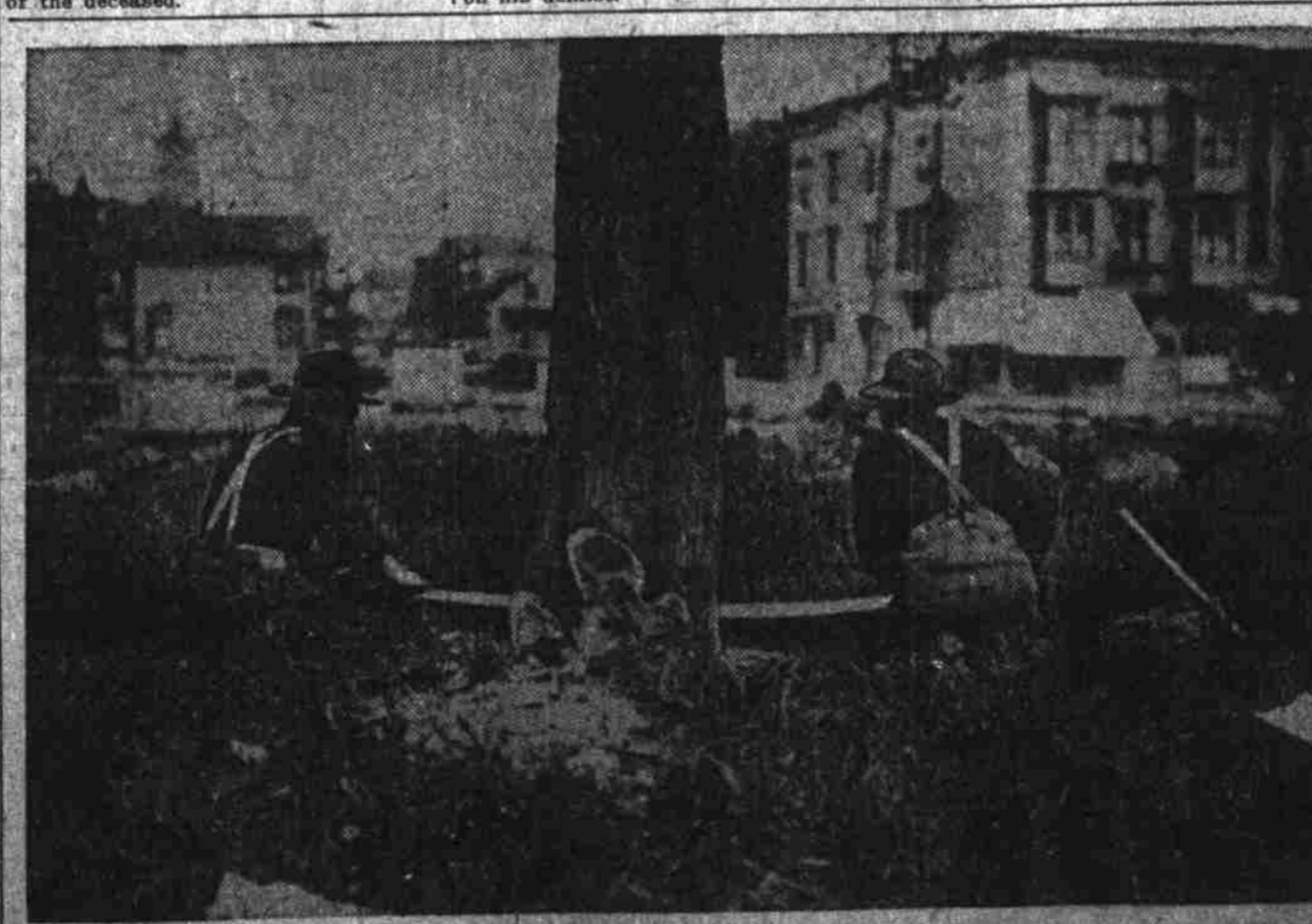
Men Working on Penneyer Block Clearing Way for Big Department Store Building.
