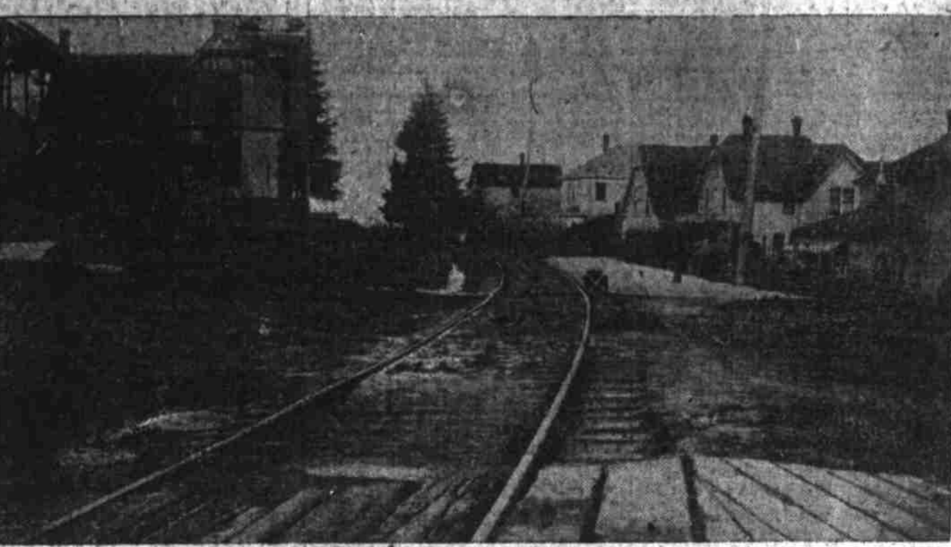
Showing Bulge in Track at Bancroft Avenue. Here the Tracks Sink Perhaps an Inch When Trains Pass.
