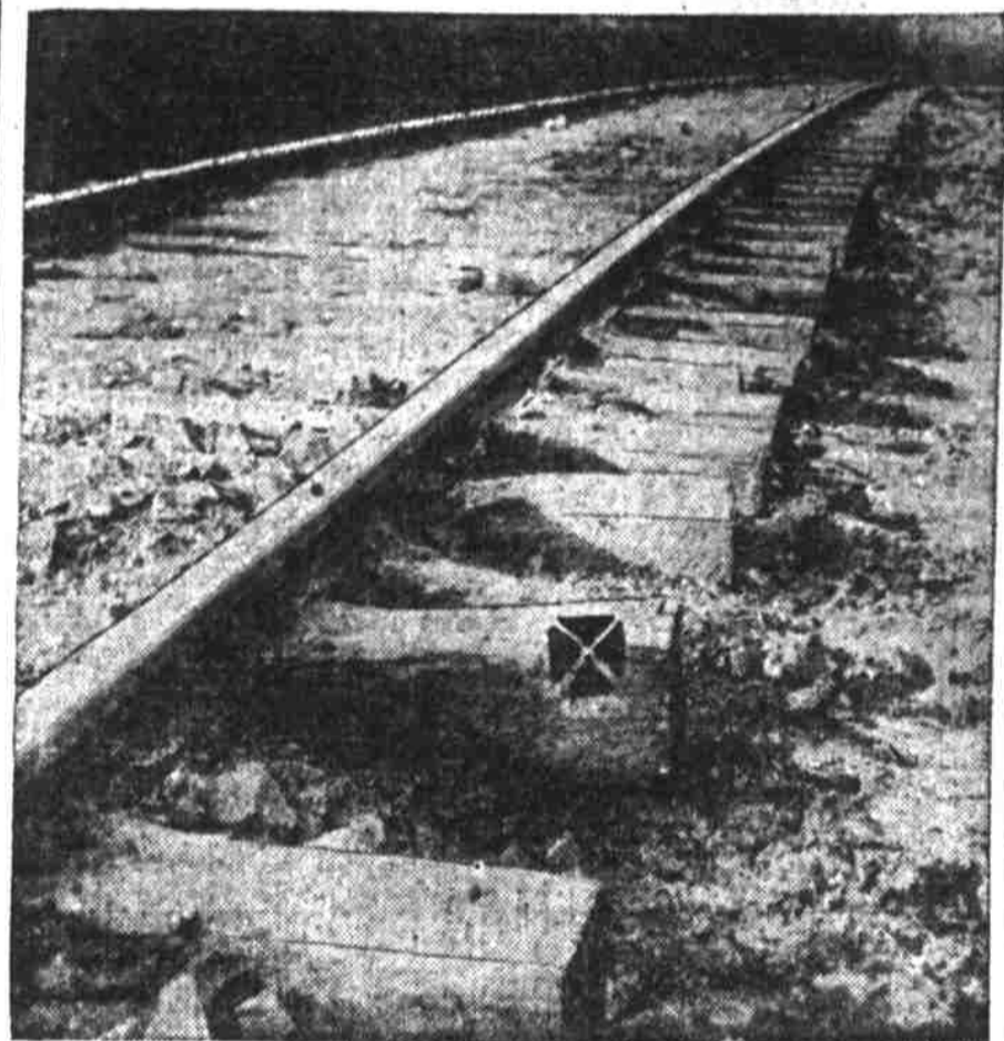
BROKEN TIE—BREAK IS UNDER TIE.
