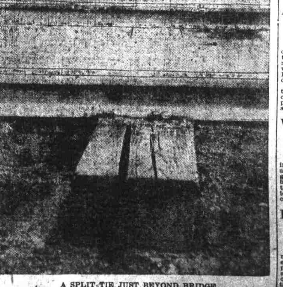
A SPLIT-TIE JUST BEYOND BRIDGE.
