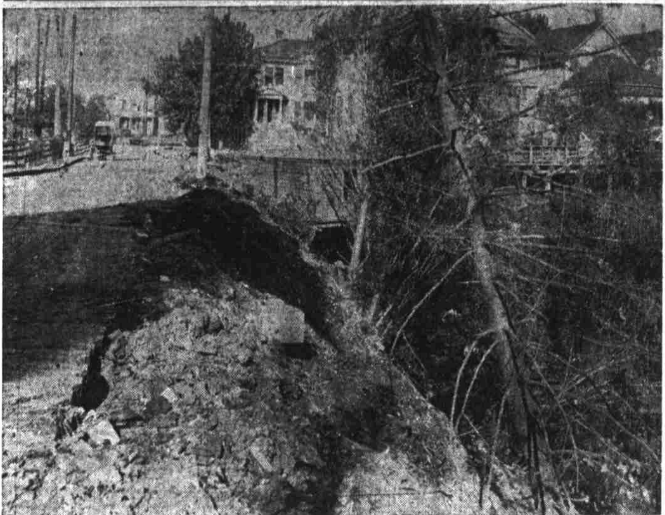
Decrepit roadway in Chapman street from which refuse is dumped by scavengers and the street sweeping department. Note the proximity of residences to this pest hole.
