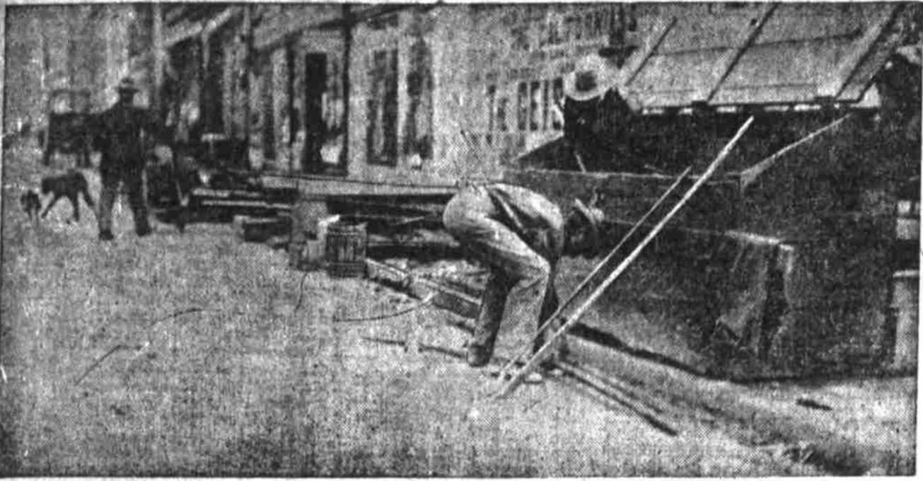
Workmen Tearing Up Rotten Sidewalk Around Disreputable Looking Kamm Property, First and Washington Streets.
