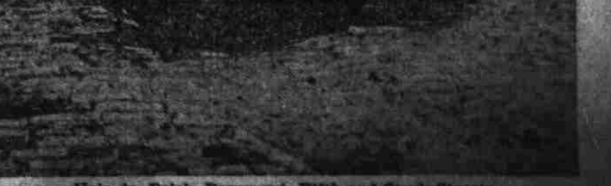
Hole in Brick Pavement, Fifth and Stark Streets
