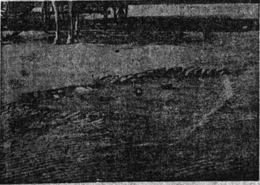
Worn Out Pavement at Fourth and Stark Streets
