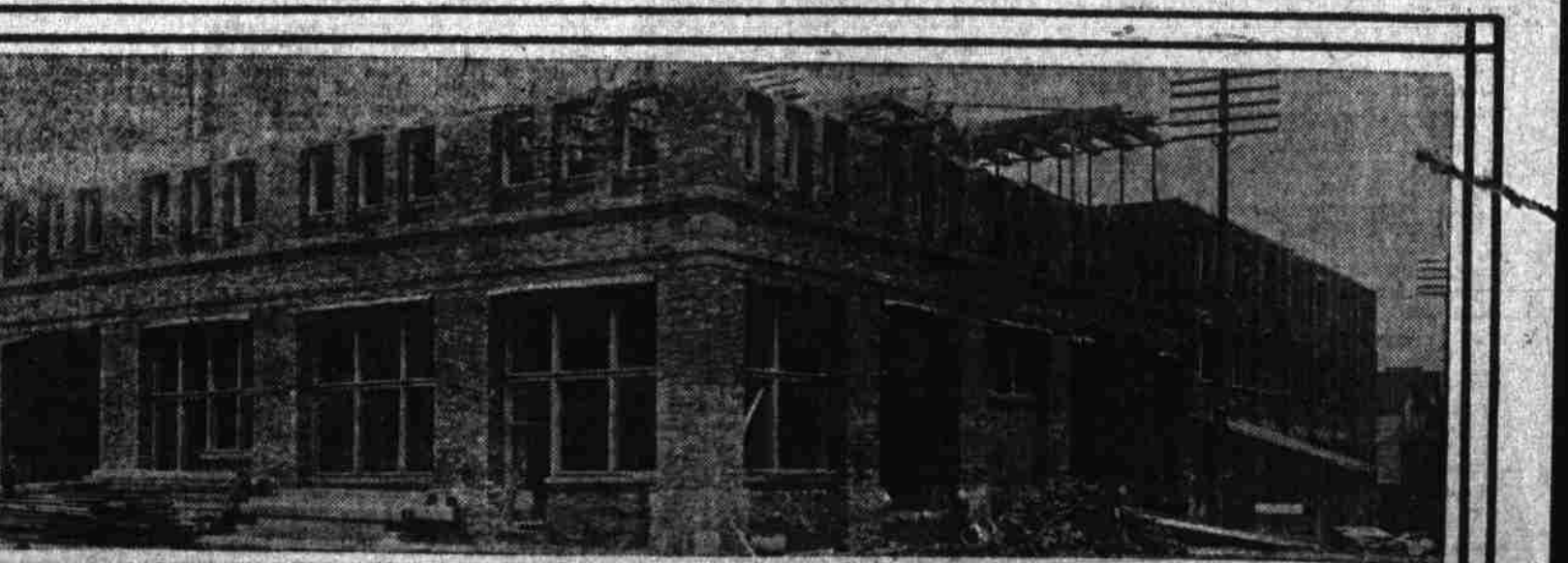
Warehouses, belonging to Joseph Simon and William Gadsby, under construction on Thirteenth, between Glisan and Hoyt.
