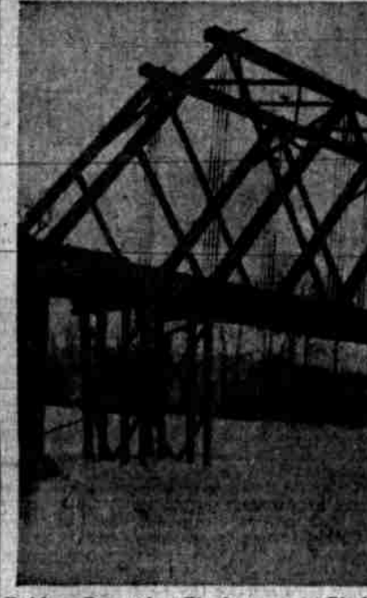
Bridge Over the Clackamas at Gladstone, Showing Three Bents Washed Out by the Flood.
