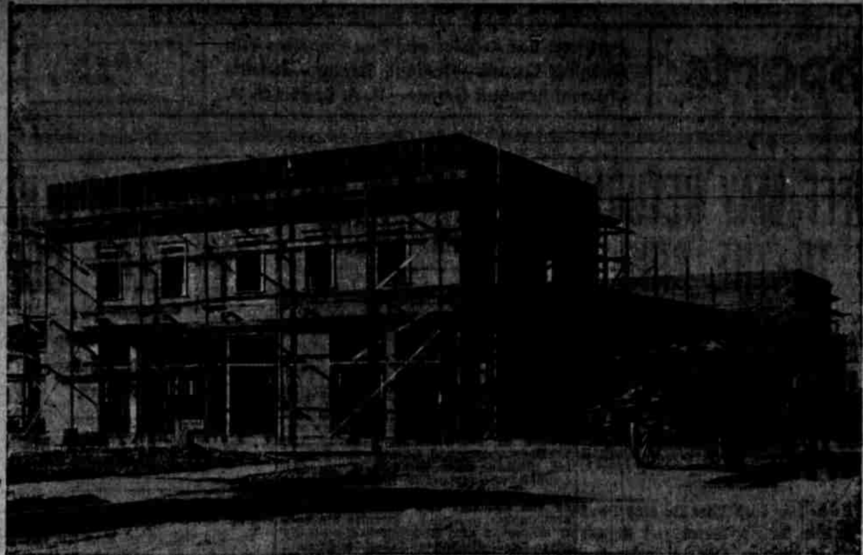
Italian Gardener's Market Building Nearing Completion at Union Avenue and East Madison Street.
