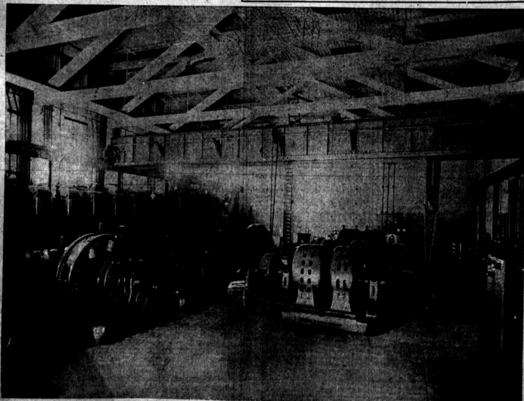
Interior of Sub-Station, Seventh and Alder Sts., where Voltage is reduced for Distribution Throughout the City, and where Alternating Current is Transformed to Direct Current for Operating Street Railways and for Service to Manufacturing Plants.
