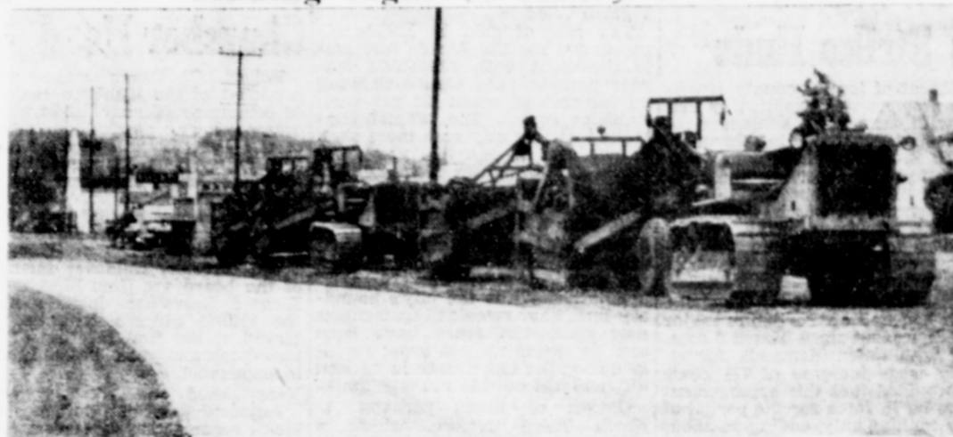
The task of widening and re-routing the West Side Pacific highway through Tigard is made easier with these machine giants. A viaduct eliminating railroad grade crossings and widening of the heavily traveled highway is included in the 99-W re-routing project.—(Cut courtesy Oregonian)
