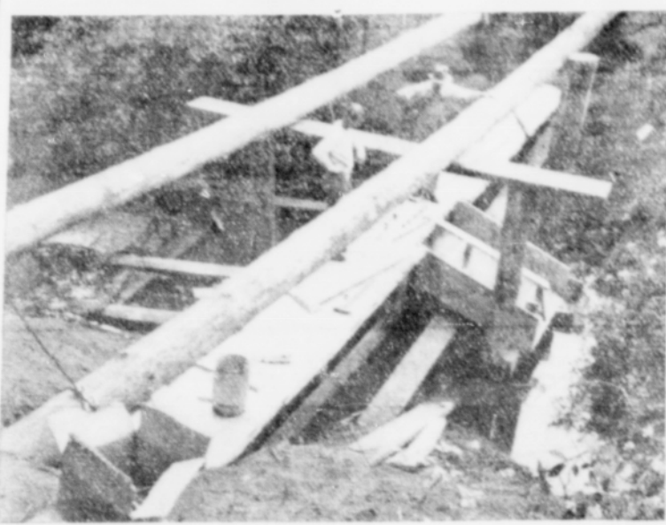
Arne Jensen (left) and Henry Chantler, in charge of construction of the McKay creek dam at Camp Ireland, inspect work progress. The chute slanting down from the dam is a fish ladder designed by Chantler. Timbers crossing the stream were used as a platform for driving piles and later removed. The dam will provide the camp with a pool for swimming and boating.
