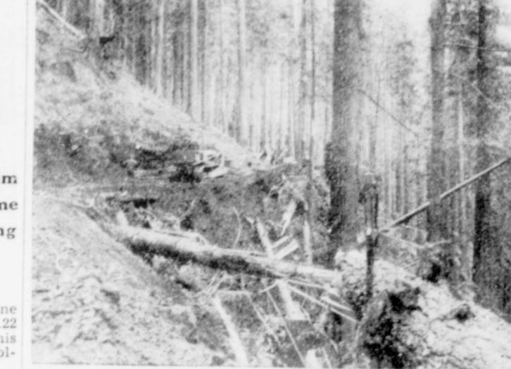
Steep slopes and rock cliffs pictured above, shows the rough nature of the terrain where Wilson river highway crews from Tillamook and Washington county are joining hands as the final few feet are cleared to open the road for passage of construction trucks between camps in the two counties, Tillamook city and Portland. Hanging 300 feet above the Devil's lake fork of the Wilson, the bulldozer thrusts and grunts as it chips away the rock. Before August 1, trucks and crew transports will be passing to and from Tillamook by way of Glenwood.
