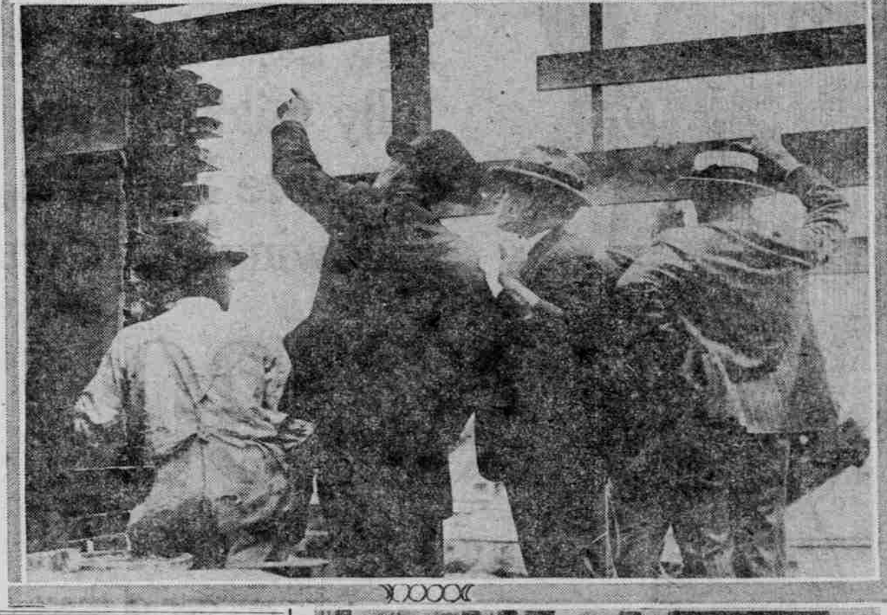
Upper-West wall of building, which was so dangerous it had to be torn down. Middle—Director Woodward (pointing finger) and Director Thomas inspecting a dangerous section of the structure. Below—This shows where rotted boards and defective brick are crumbling to pieces.
