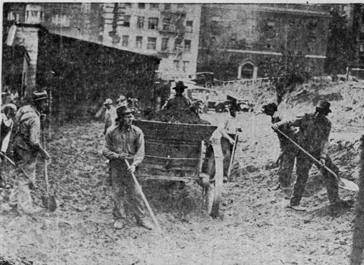
SNAPPED AT NINETEENTH AND COUCH STREETS LAST WEEK AS GRADING TEAMS BEGAN WORK. This new addition will add a two-story brick and concrete building, 60 feet wide by 200 feet long...
