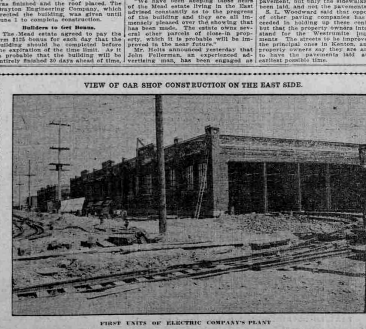
FIRST UNITS OF ELECTRIC COMPANY'S PLANT
