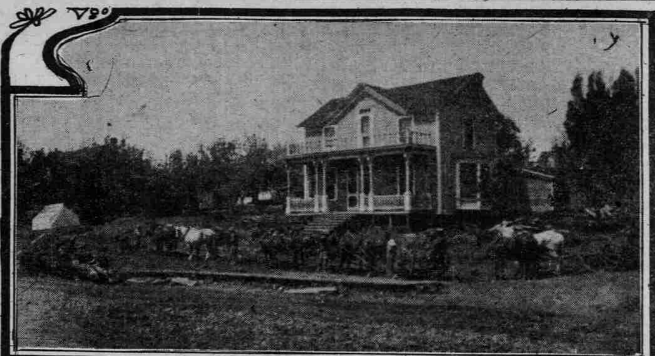
EXCAVATION FOR HAMMAR BUILDING NORTH SIDE OF MAIN BETWEEN SECOND AND THIRD.
