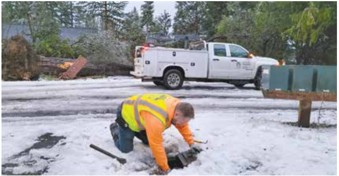
Water Bureau employee searches for the source of a broken water line (Photo courtesy of City of Portland)
