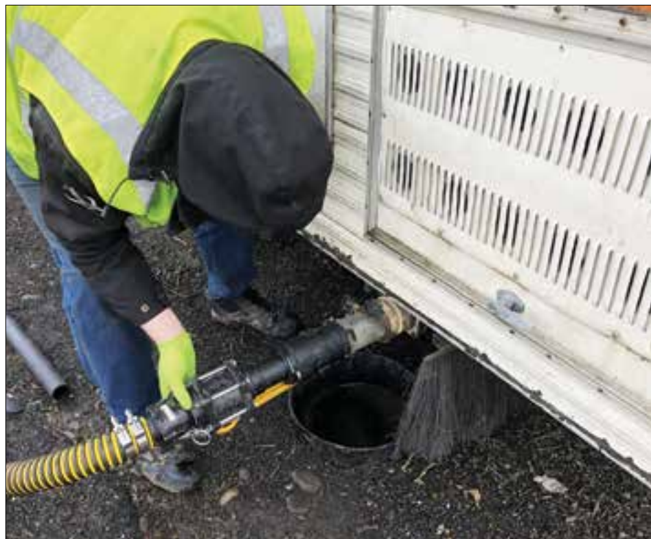
Portland Environmental Services launches a pilot pump out program to help houseless people living in a recreational vehicle to safely dispose of human waste and prevent environmental contamination.
