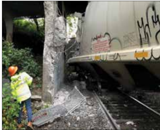
A Union Pacific freight train derailed early Tuesday in north Portland and one of the cars jammed up against an overpass on North Lombard Street. (Photo by Portland Bureau of Transportation)
