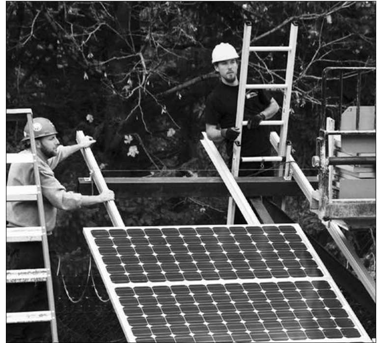
Solar panels are lifted into place for the Oregon Solar Highway Demonstration Project. The archive photo is from the Oregon Department of Transportation.
