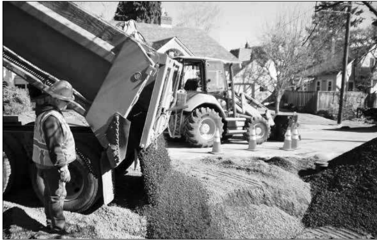
PHOTO BY DANNY PETERSON/ THE PORTLAND OBSERVER A city of Portland construction crew on Monday fills a whole left in the street caused by a broken water main, a major supply line that caused flooding, evacuations and a power outage of over 10,000 homes. Portland Water Bureau crew worked around the clock from when the pipe burst Saturday morning until a replacement was set and buried Monday morning.
