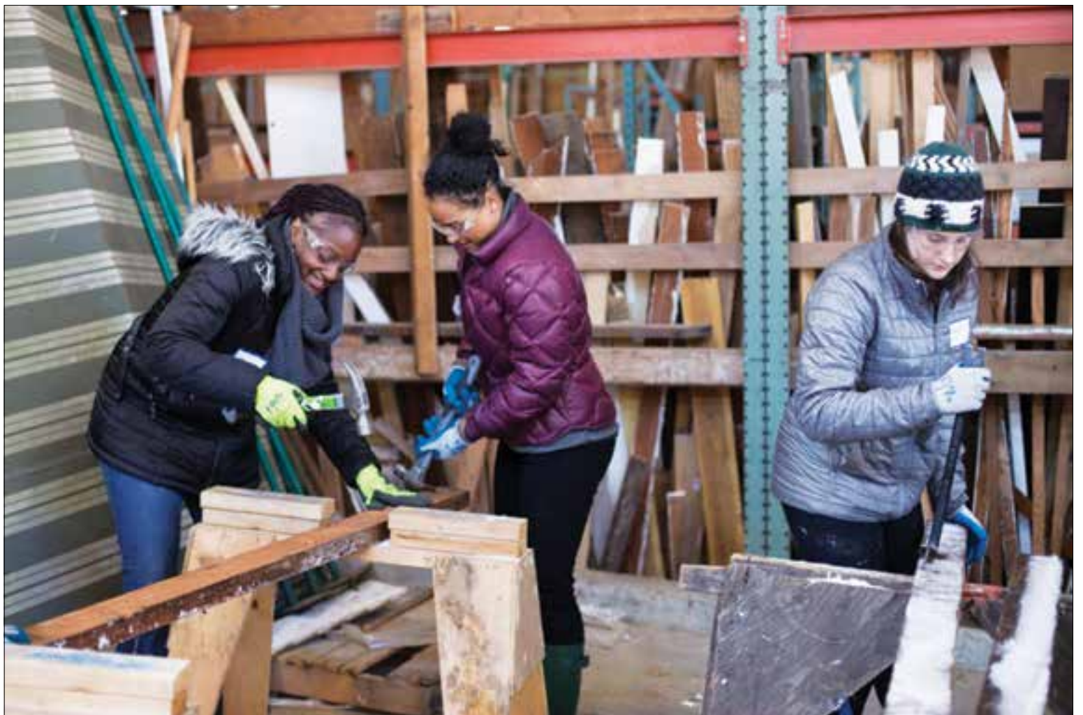
Volunteers at the non-profit Rebuilding Center on North Mississippi Avenue honor Dr. Martin Luther King Jr. and his legacy by preparing materials for home repairs that are affordable for everyone. Sponsored by the United Way, nearly 2,000 volunteer opportunities will be part of this weekend’s annual MLK Weekend of Service.
