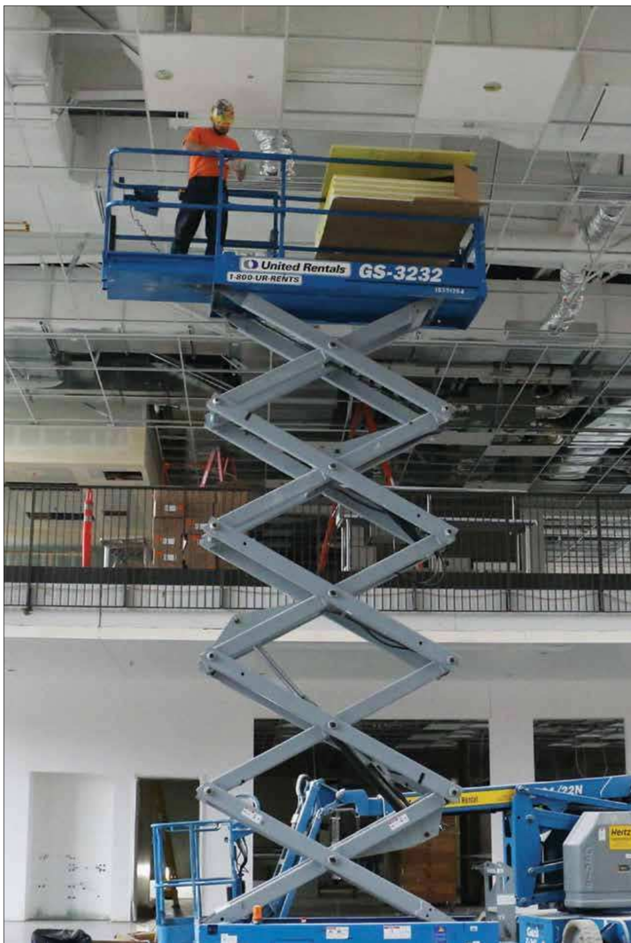
A crewmember from Skanska USA, the construction firm contracted by Portland Public Schools to complete the renovation of Franklin High School, works to remodel and modernize the historic building's central atrium. Franklin High School was originally built in 1917.
