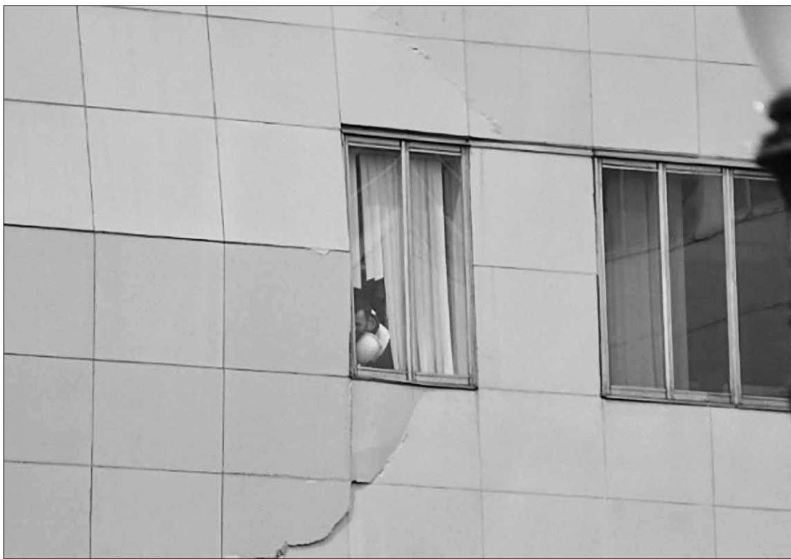
A KOIN-TV photo shows the large bulge and crack found Tuesday on a 10-story office building in downtown Portland Tuesday.
