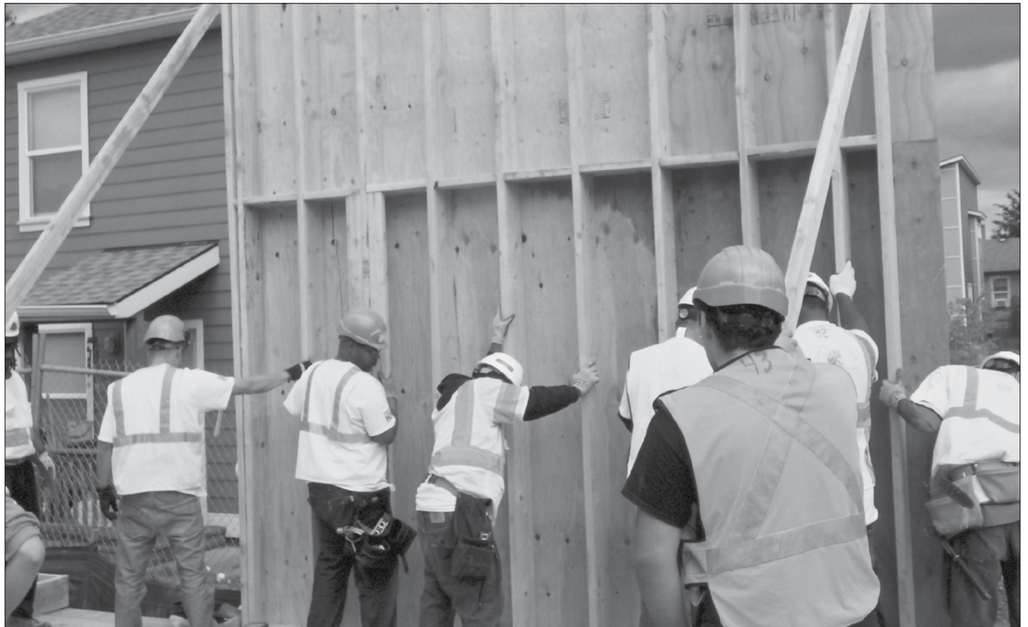
A free 9 week pre-apprenticeship training program offers 180 hours of classes and hands-on training for jobs in construction.
