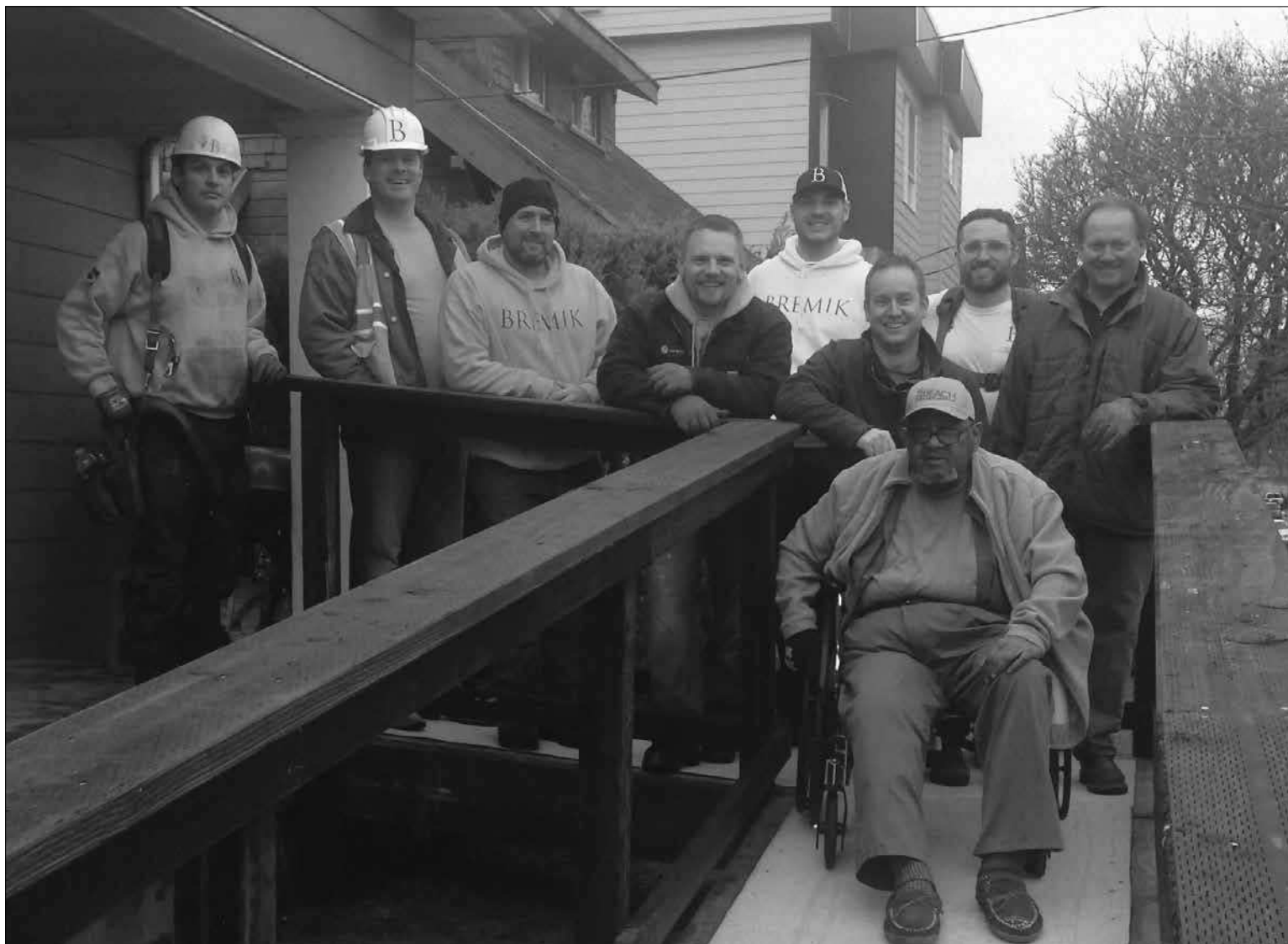
Critical home repairs, including a wheel chair/accessibility ramp, give long-time resident Charles Adams the ability to stay in his inner northeast Portland home. Adams, 68, is pictured in front of the crew that recently performed some of the needed construction.
