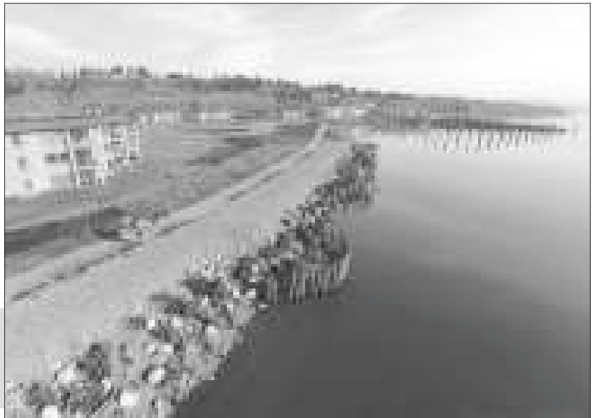
An aerial view of Vancouver's Waterfront Renaissance Trail as repairs near completion.
