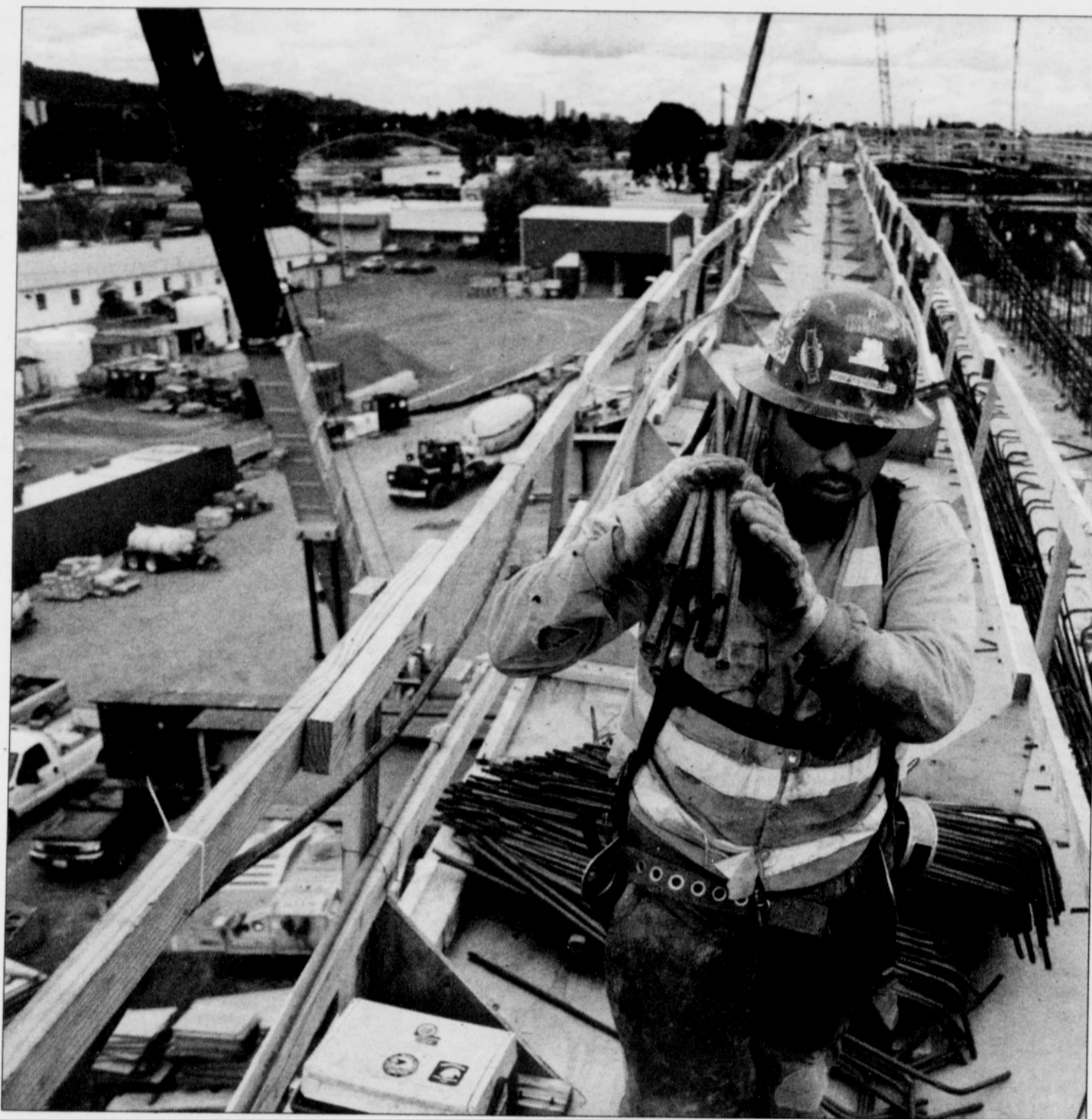
TriMet officials reported a milestone with construction of the Portland-Milwaukie Light Rail Line and its creation of 10,000 jobs so far and a record $153 million in contracts to minority, women and other disadvantaged business firms.
