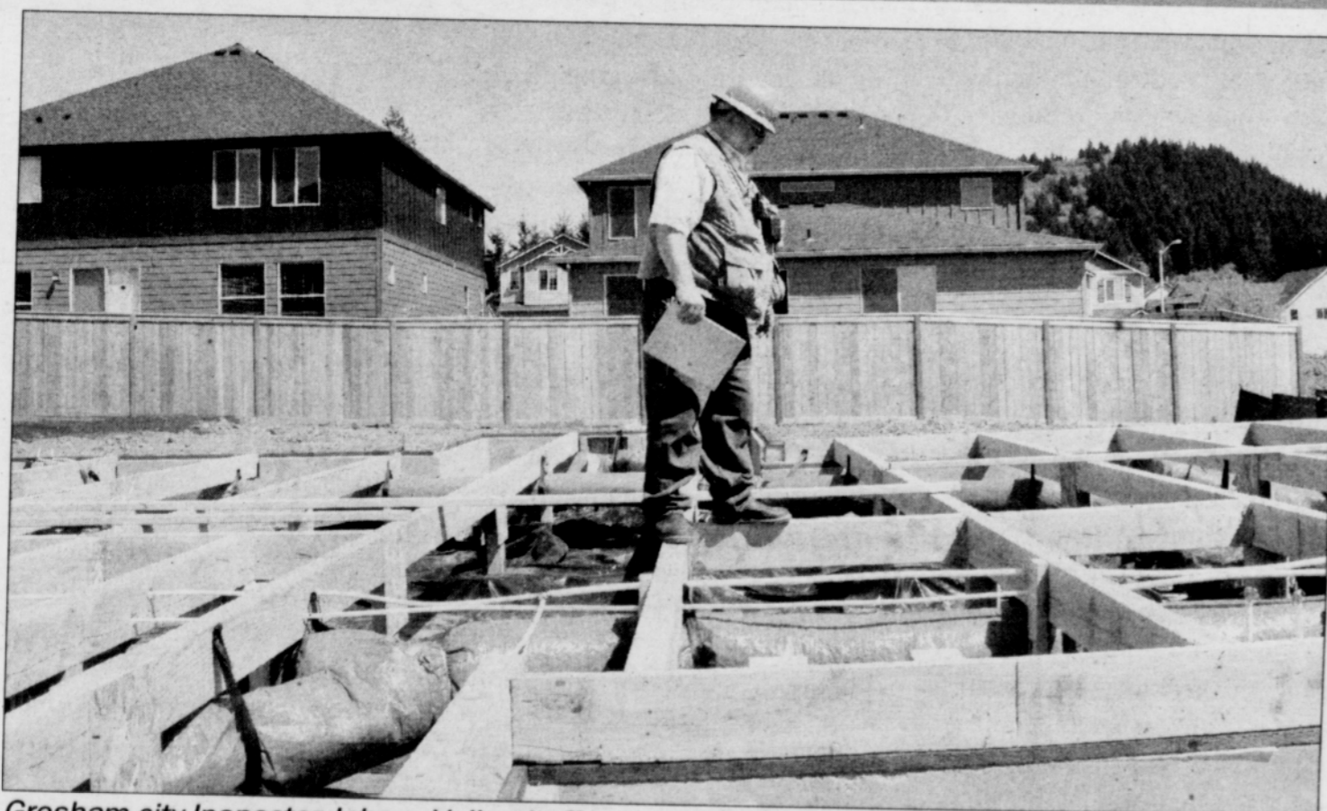
Gresham city Inspector Johnny Vollendroff inspects a new home under construction with the use of students at the ACE Academy for Architecture.
