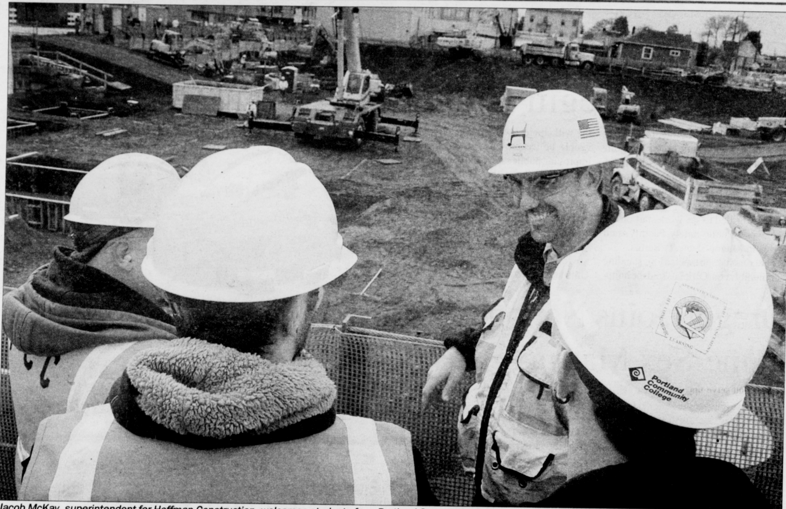
Jacob McKay, superintendent for Hoffman Construction, welcomes students from Portland Community College's trades preparation class to the Portland Community College Cascade Campus where two buildings and an underground parking garage is be constructed along North Albina Avenue.
