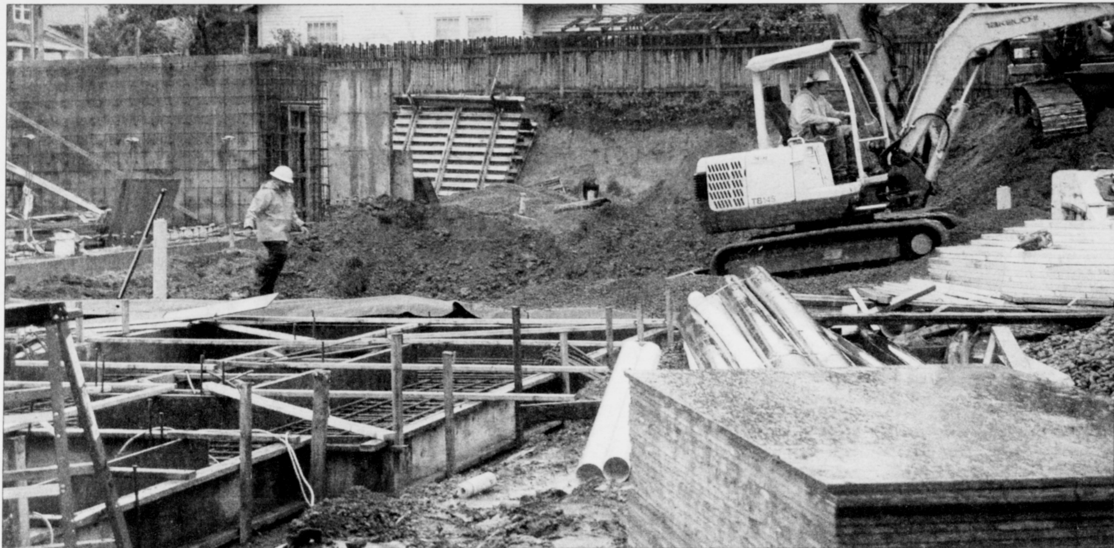
Construction of a new apartment complex for up to 50 low and moderate income residents is underway on the corner of Northeast Martin Luther King Boulevard and Cook Street in the Eliot Neighborhood.
