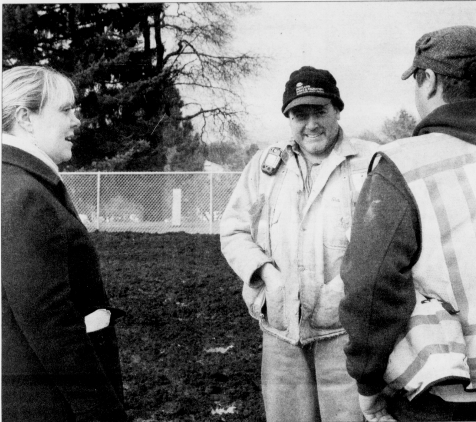
PHOTO BY MINDY COOPER/THE PORTLAND OBSERVER Community Gardens Program Coordinator Laura Niemi and Parks and Recreation employees Shane Crone and Earl Straley oversee the construction of a community garden in northeast Portland.
