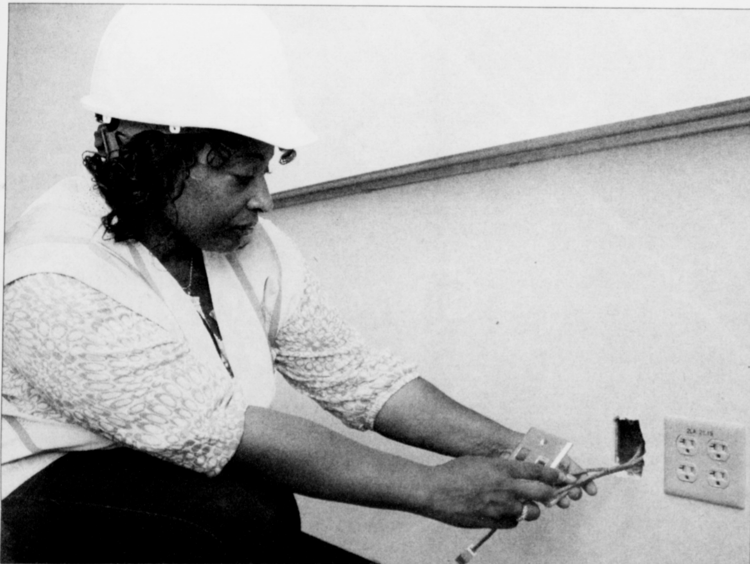
Sharon Maxwell-Hendricks, the locally-owned owner of the Boanerges Group, a contracting agency with 50 employees, inspects remodeling work her firm completed on the Cascade Campus of Portland Community College in north Portland.
