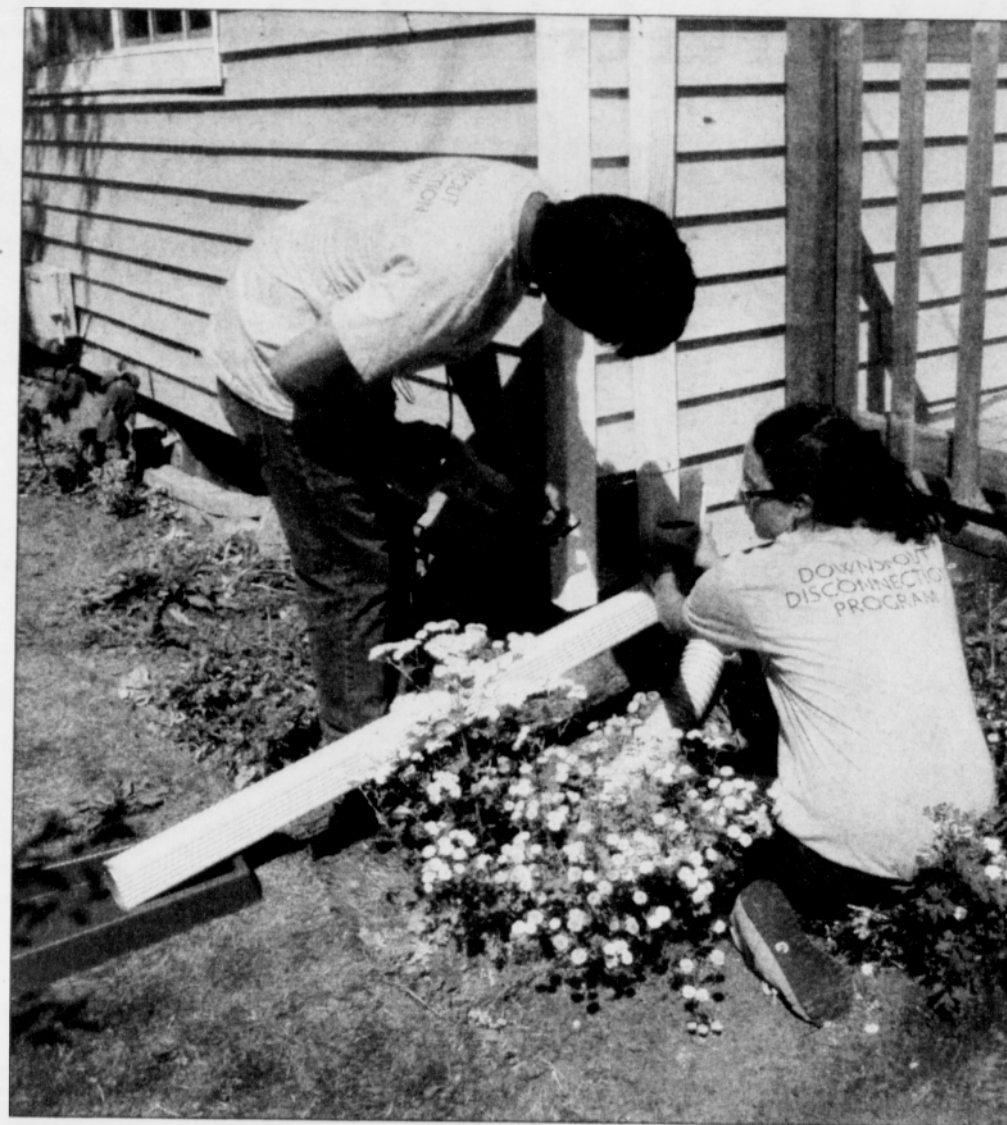
Gresham volunteers disconnect a home's downspout through a program to help prevent water pollution run off.
