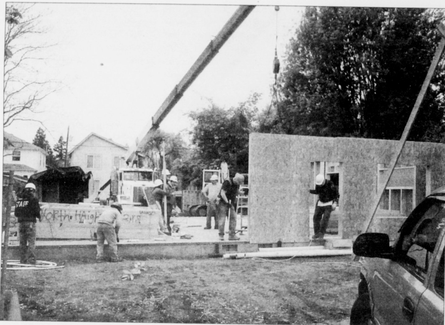
Wall panels that were constructed offsite are installed at a home construction site in north Portland for Habitat for Humanity. The newest technology replaces site framing and has fewer environmental impacts by reducing waste and theft.
