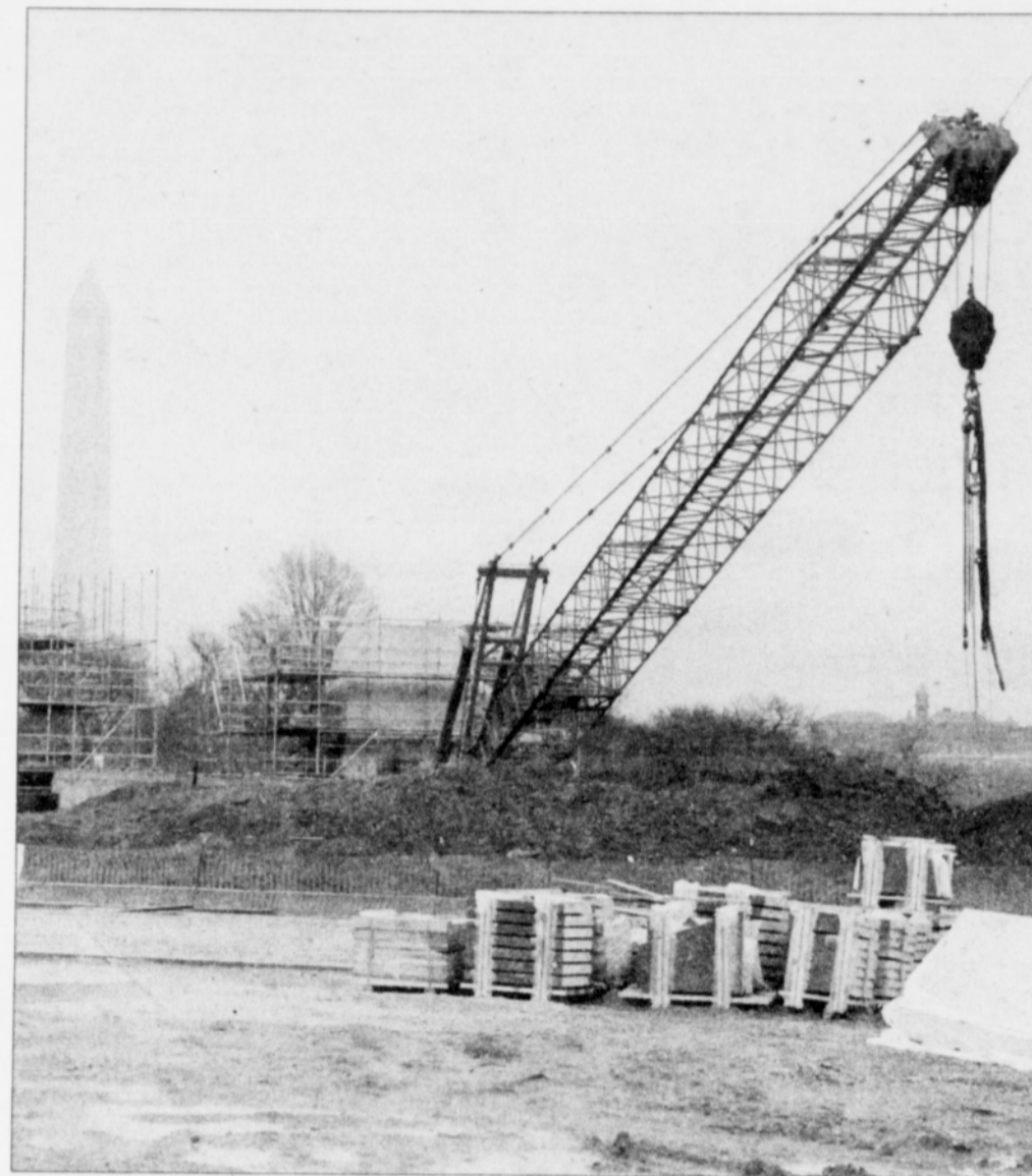
Construction is underway on the Martin Luther King Jr. National Memorial on the National Mall in Washington, D.C.
