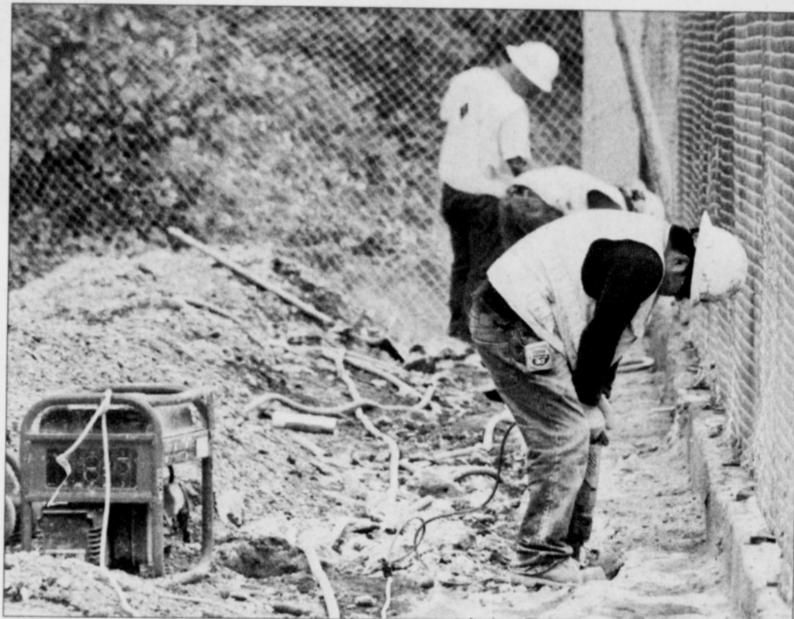
Julio Rodriguez of R&R General Contractors works on the Civic Drive MAX station in Gresham.
